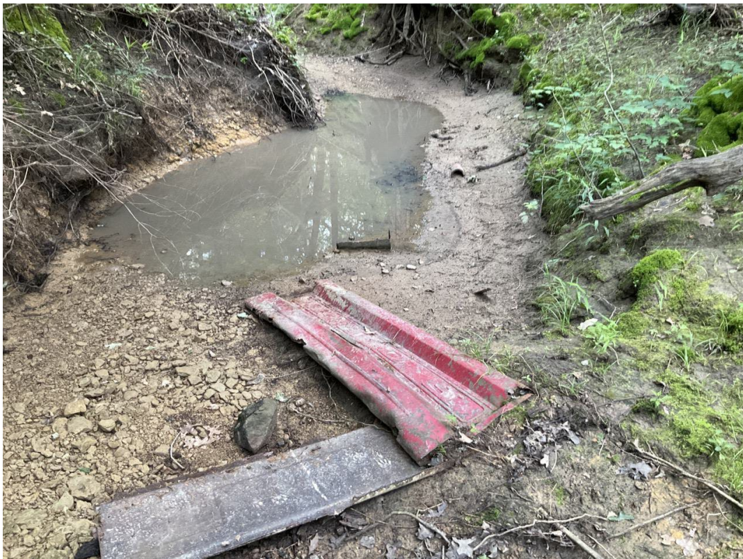
Photo 08: Metal debris in stream.
